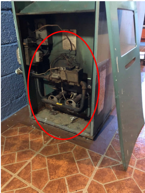
Scorched Cabinet Interior
